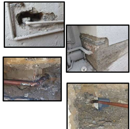
Work done on Unit 85, water leak on outside due to aged and rotten pipes and corrosion
